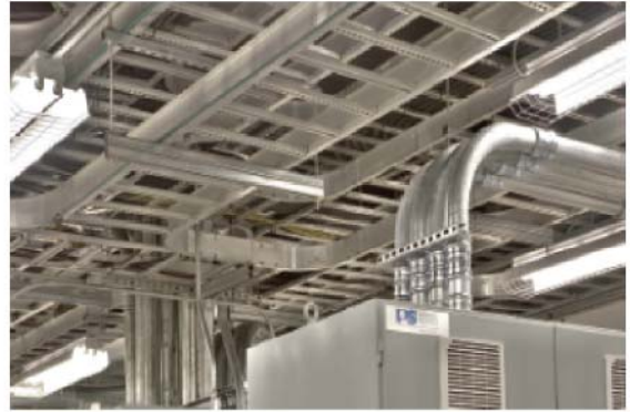
Solutions for Data Center
